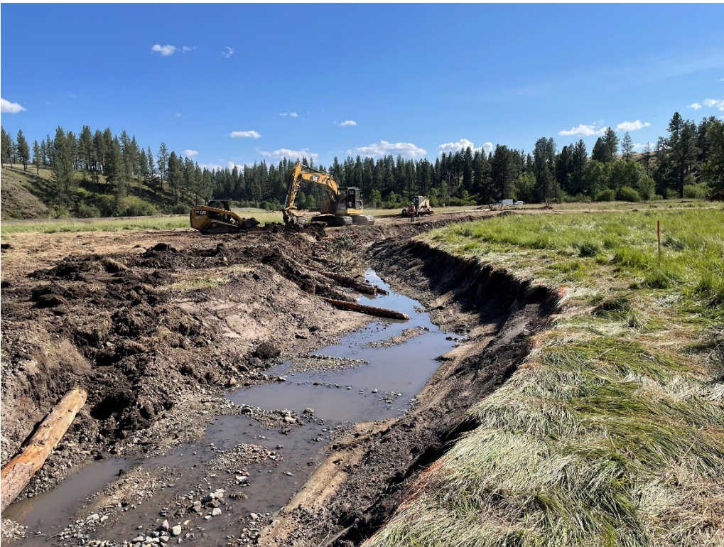
Figures 3 and 4. ODFW staff directing large wood placement in the recently constructed side channel.
