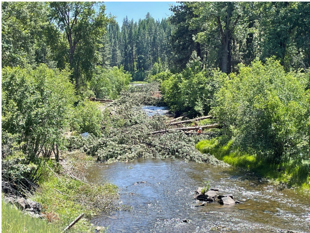
Figures 1 and 2. Installation of Large Wood Accumulations using a Vertol 107 and view upstream of placed wood before substrate augmentation.
