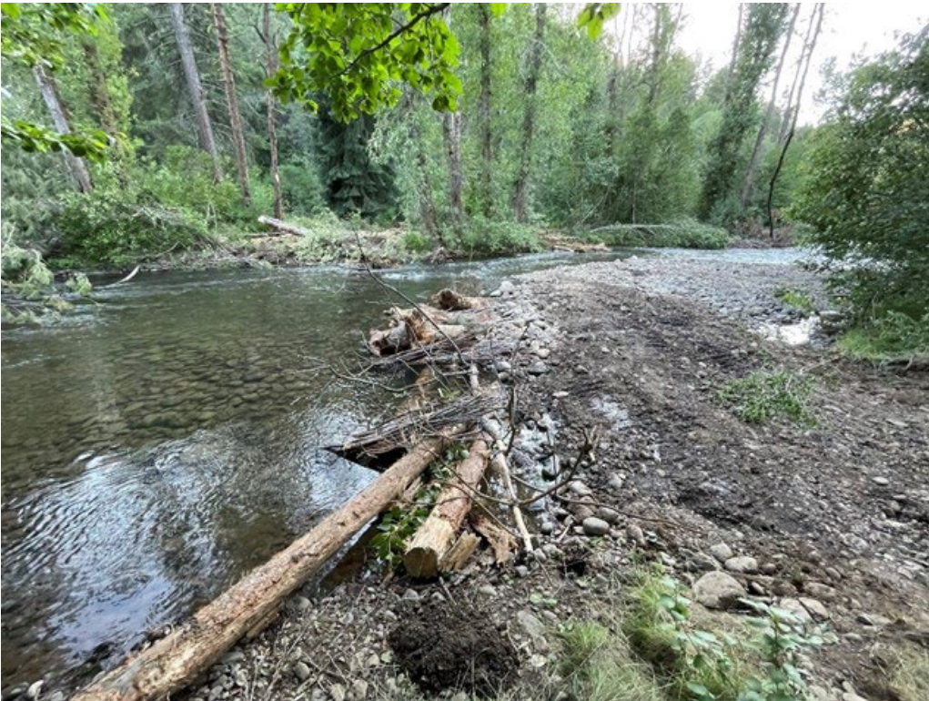
Figures 5 and 6. Construction of Pool-Bar-Wood complex and built Pool-Bar-Wood complex. Note width to depth reduction.
