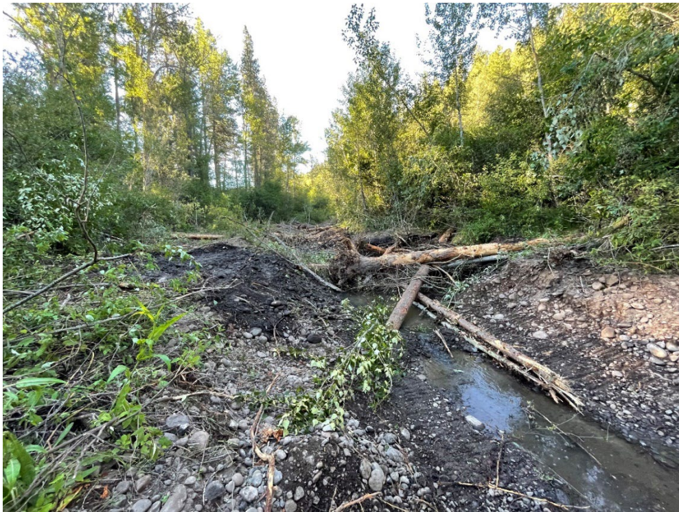
Figures 1 and 2. Installation of LWD structure in newly constructed side channel and the completed side channel and large wood structures before activation.
